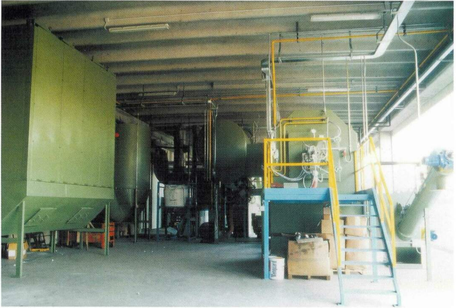
From left: bag filter, reactor, adsorbent batching, post-combustion, rotary kiln, ash discharge
