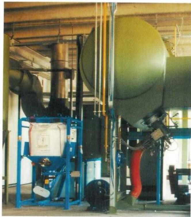
Post-combustion chamber with burner, dosing system
