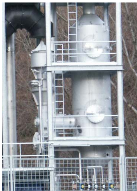
Wet venturi and scrubber
