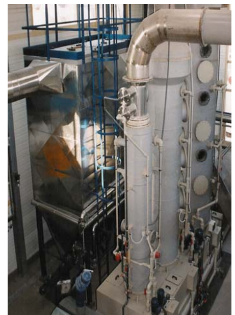
Combined wet and dry system
